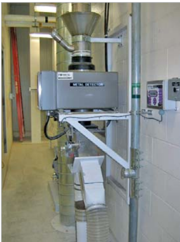
One of five Phantom Gravity metal detectors used to detect metals in free-flowing oat products before packaging.
